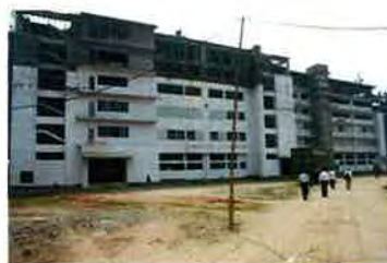
The new plant under construction. Expansion is made at full speed to meet the yearly growth of the business.
